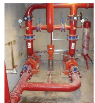
Bomba Jockey Bomba principal Bomba auxiliar
